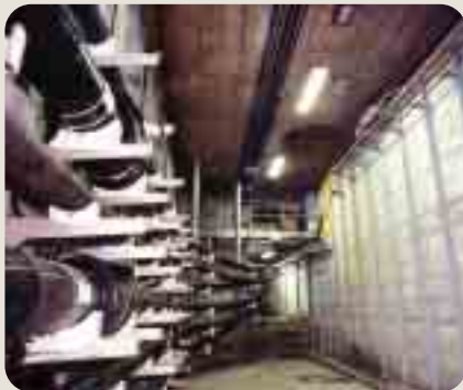
High-voltage power cable in a tunnel
